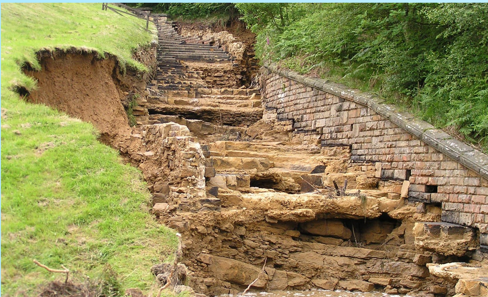
Masonry Stepped Spillway Failure Due to Plucking Damage
