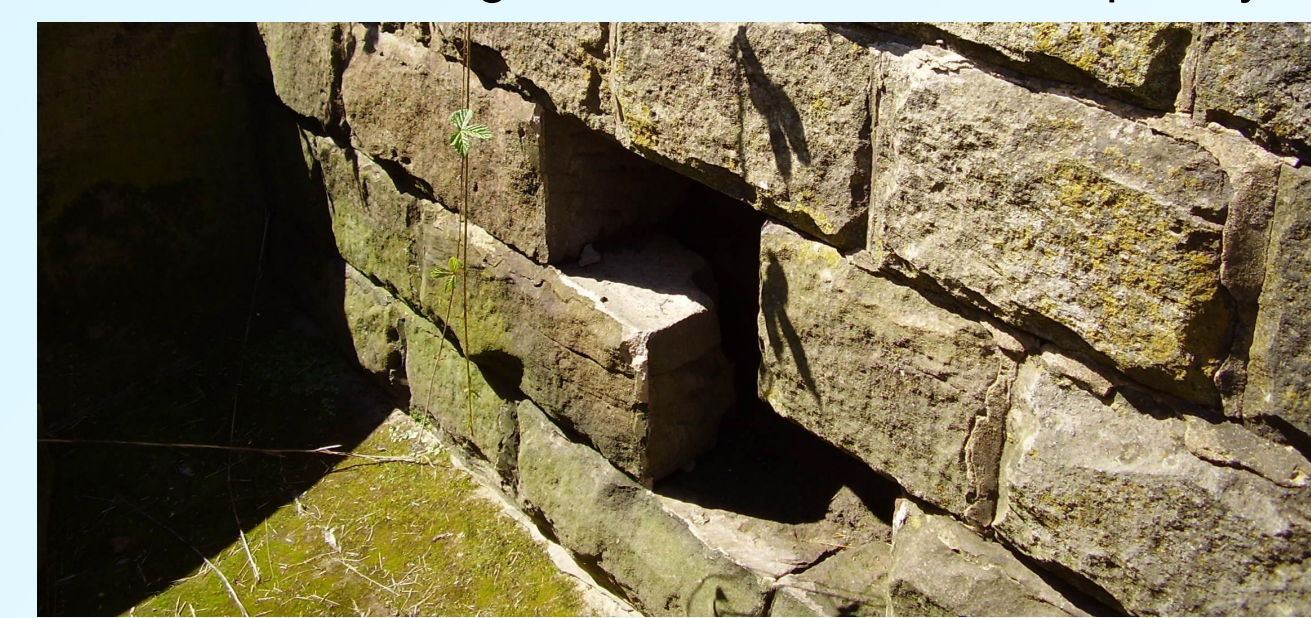
Plucking Damage on a masonry stepped spillway
